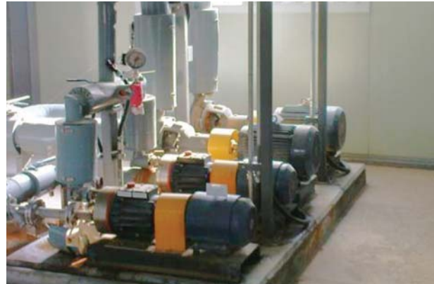
Figure 5. Installing seal-less Hydra-Cell pumps removed leak problem and halved energy use at Seonam.
