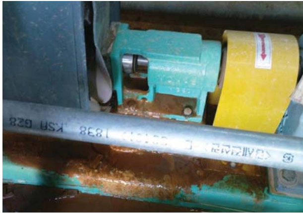
Figure 4. Seal leaks lower efficiency and waste power. (Water treatment plant, Seonam).
